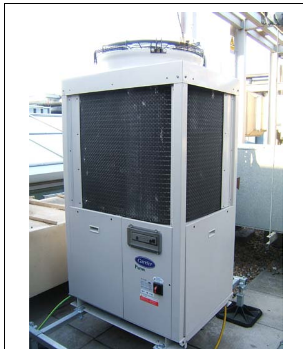
Photo 6: It may not look much but DECC's IT chiller, installed in December 2010, is expected to yield significant carbon savings.
